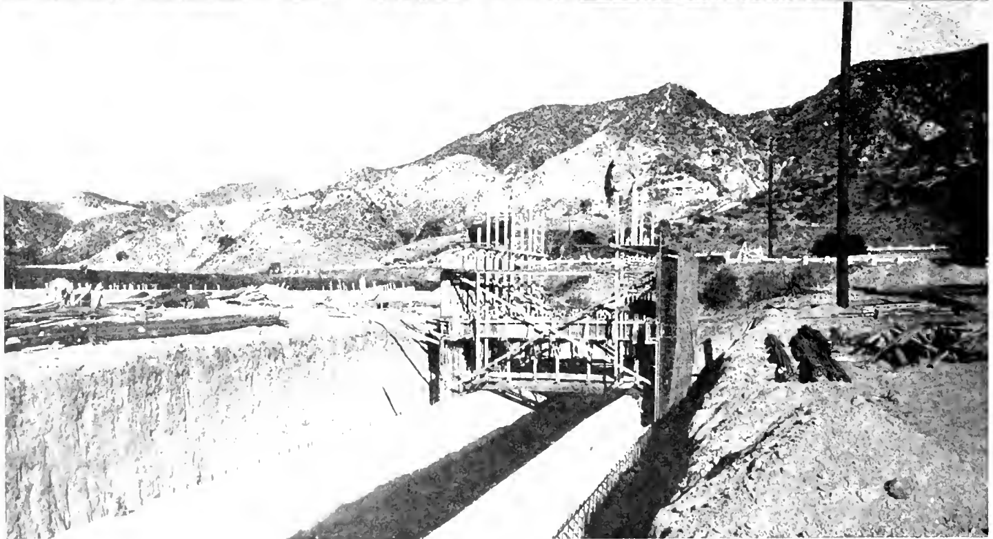
UPPER Looking southeasterly, showing portion of half-million-yard fill under construction in Weldon Canyon. LOWER Looking northeasterly along Owens Valley- Los Angeles open channel aqueduct, showing special design, reinforced concrete bridge construction to permit passing of freeway over the aqueduct.
